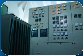
ELECTRICAL DISTRIBUTION BOARDS
